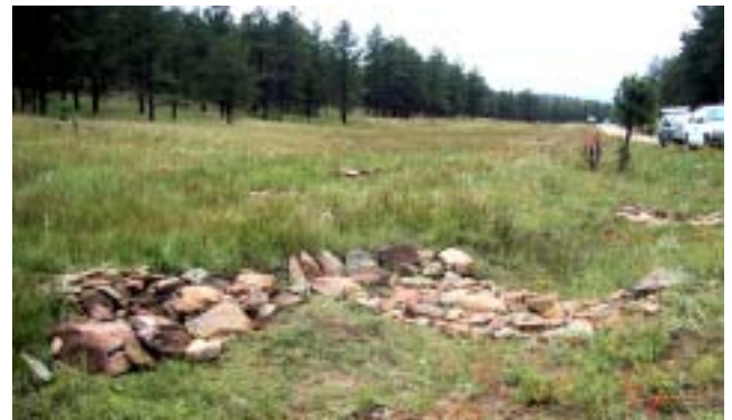
Many loads of rock went into building this erosion-defying structure in Lookout Canyon on the east side of Valle Vidal.
