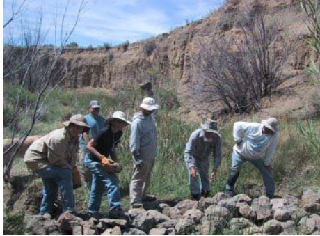
Sunday, working on the BIG rock dam: (l to r) Patricia Hester, John Perea, Glenda Muirhead, Michael Scialdone, Bill Zeedyk, Gene Tatum.
