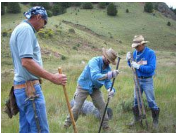
“Chip”, Hamish Thomson and Dennis Muirhead deepen a fence-post hole with shovel, rock bar, and posthole digger, as part of a fencing enclosure on Comanche Creek.
