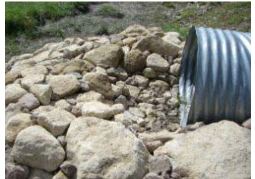
One of Sunday's projects: Diversion/overflow rock structure at culvert mouth to help spread upland drainage under the road to the meadow on the other side.
